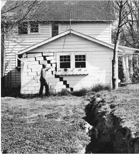
Paying attention to soil interpretations can help builders and landowners avoid this kind of disaster. Soil slippage and swelling caused this house to break apart.
